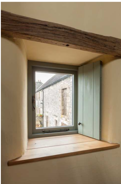
Figure 5 Insulated lime plaster walls conserve the internal appearance of the historic building whilst conserving energy. Home made internal shutters also conserve energy.
