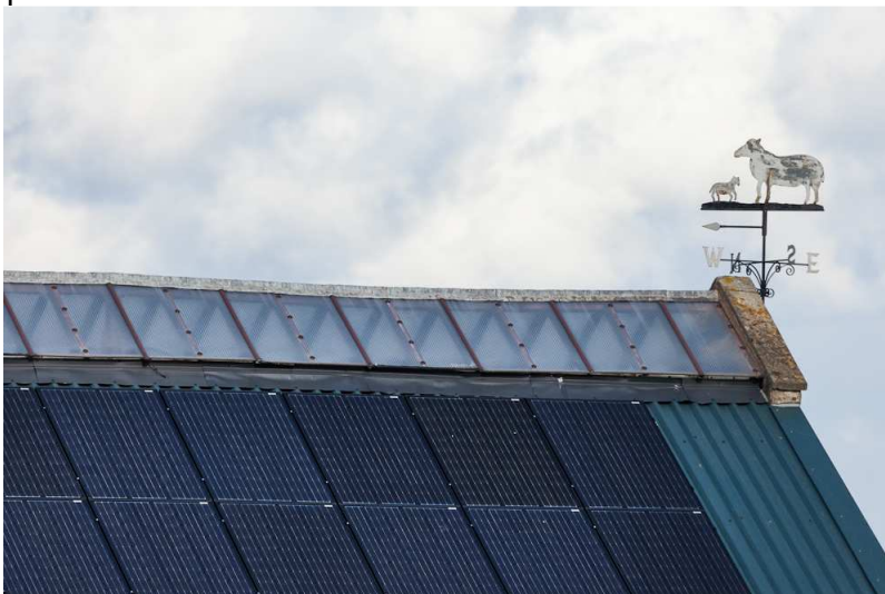
Photo 8 Photovoltaic panels on patent glazed roof.
