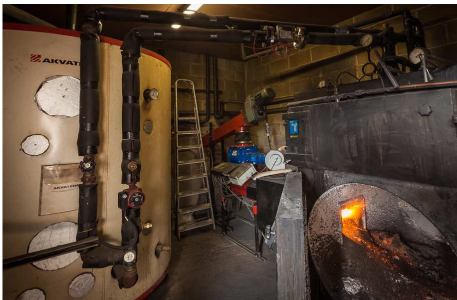
Photo 16. Mini district heating system at Beechenhill Farm
