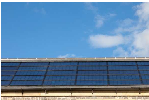
Figure 2 Solar photovoltaic panels
